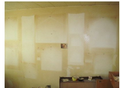
Secondhand smoke residue is obvious after pictures are removed
