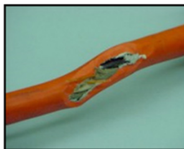
Image 2. Frayed Extension Cord
